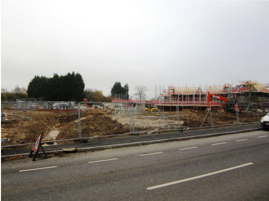
Plate 9: View of Somerfield Barn Complex from the A20 with ongoing development in the forefront – facing SW
