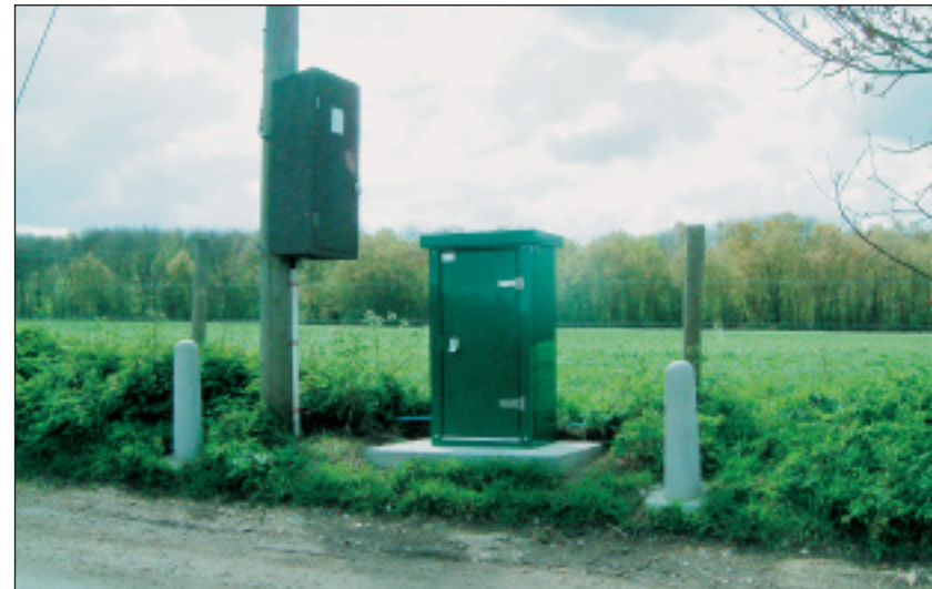
Far left: Poorly sited telecommunications mast
