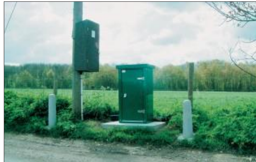
Far left: Poorly sited telecommunications mast
