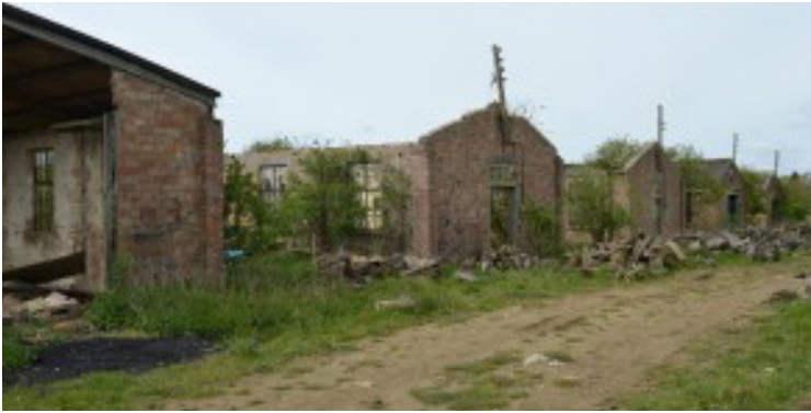
Former Barracks Huts (35). Note: this is outside the application boundary but within the wider framework masterplan area.
