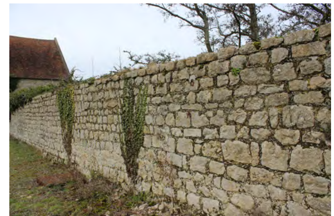
Figure 116: Detail of stone wall bounding the north side of the area to the east of the barns
