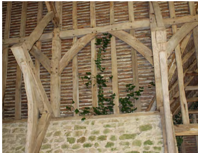
Figure 111: Detail of the roof structure towards the north end of the barn showing encroaching ivy
