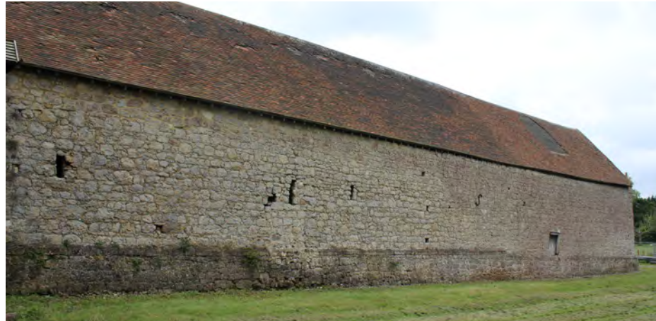
Figure 87: View of the north elevation looking south-west showing later ventilation slits and openings
