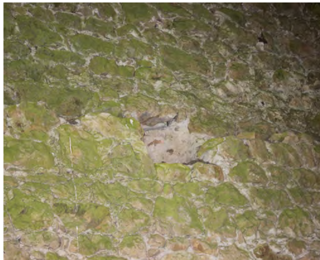
Figure 92: A representative socket for supporting a tiebeam indicating the present of an original first floor in the west room
