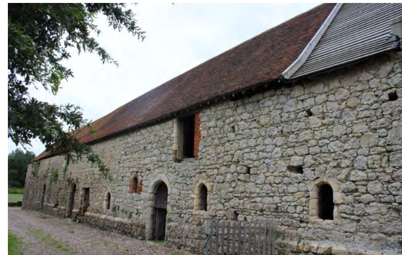
Figure 85: View of the south elevation looking north-west showing piecemeal fenestration and a section of untiled roof
