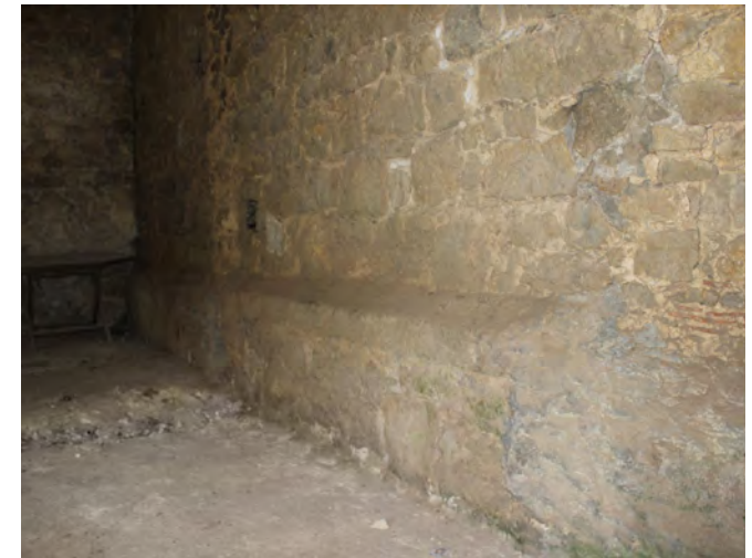
Figure 112: Detail of the east elevation of the east-west barn, featuring its distinctive stone plinth, projecting into the later north-south barn. This is a reminder of the construction sequence of the two barns, indicating the north-south barn was added on to the end of the earlier east-west barn.
