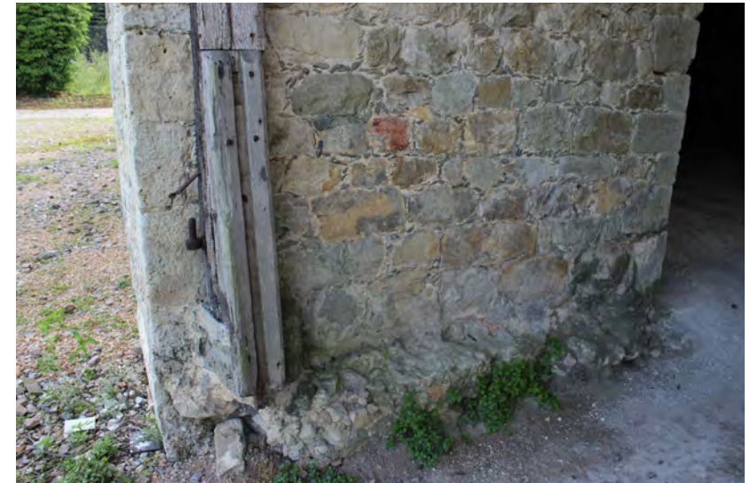
Figure 104: Detail showing a representative grooved doorway feature or 'leap' where boards slotted to stop grain being blown out of the barn
