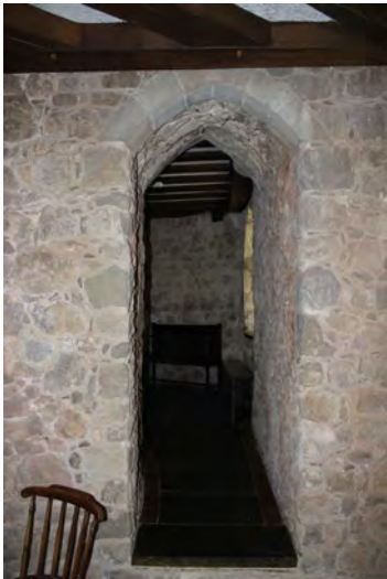
Figure 65: Arched passage from the main function space to the north-east tower and former bakehouse
