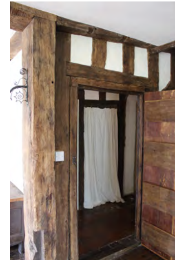
Figure 53: Remains of timber-framing at ground floor level in the main (south) range
