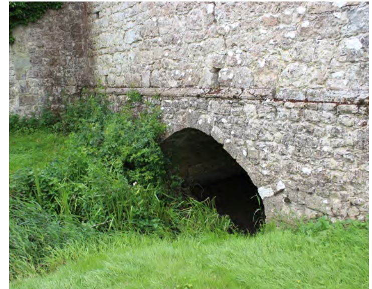
Figure 107: Detail of the arched stone culvert at the north end of the barn
