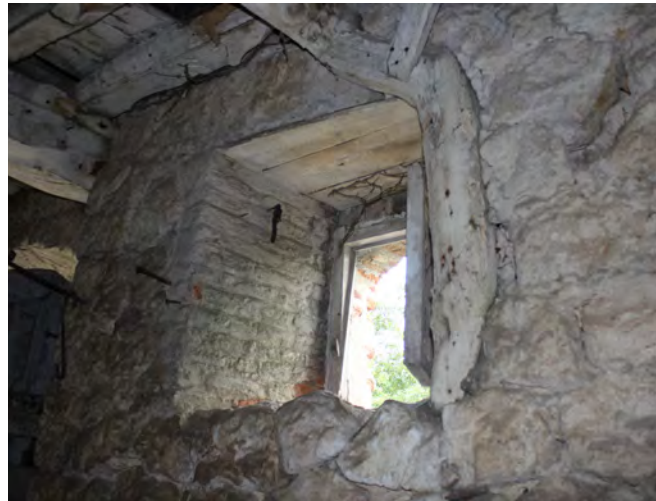
Figure 98: Internal view of a later window as indicated by the brick and timber construction around the opening
