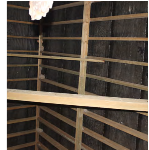
Figure 100: Detail of the largely modern roof structure at the east end of the building
