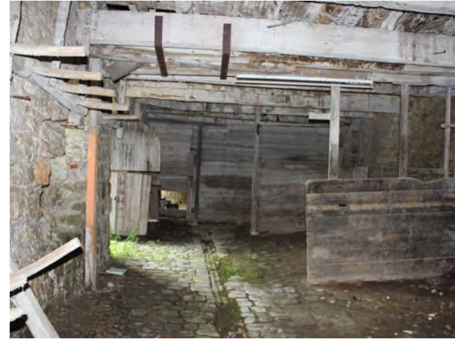
Figure 96: View of the east room with stone guttering in the floor and timber partitions evidencing former use as accommodation for livestock
