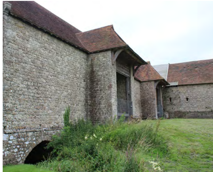
Figure 106: View of the west elevation looking south showing the arched stone culvert at the north end of the barn
