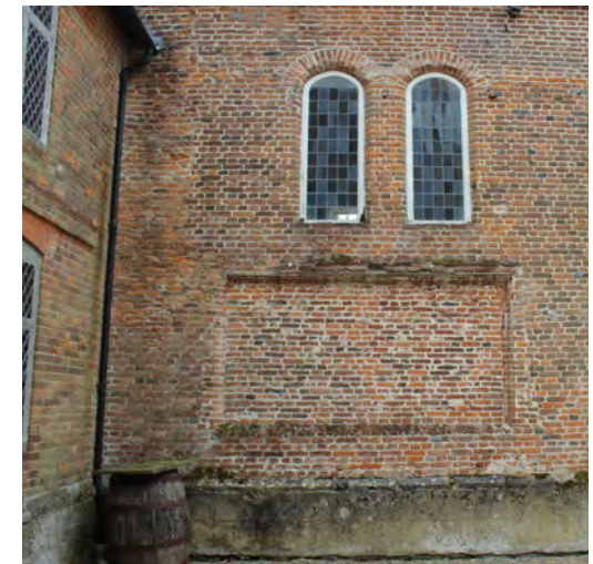
Figure 45: Detail of the north elevation of the main range showing the 16th century paired round-headed windows and blocked rectangular opening below
