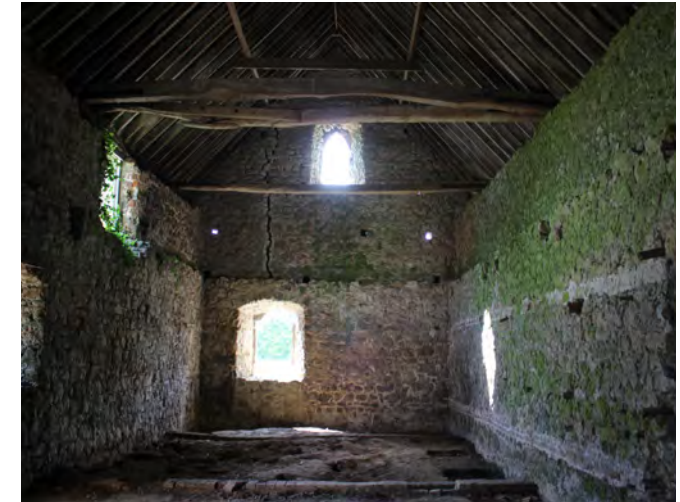
Figure 91: View of the west room looking east showing historic and later openings and a crack in the west gable
