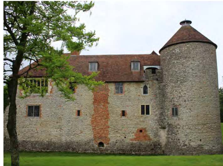
Figure 46: View of the east elevation of the rear wing which is characterised by its tall 14th century coursed ragstone curtain wall with later brick interventions
