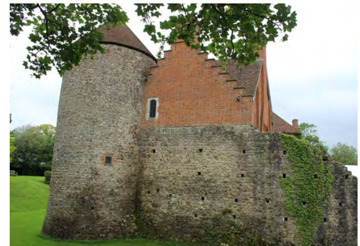
Figure 49: View of the north-east tower from the north showing an original window on the left and a modified window on the right
