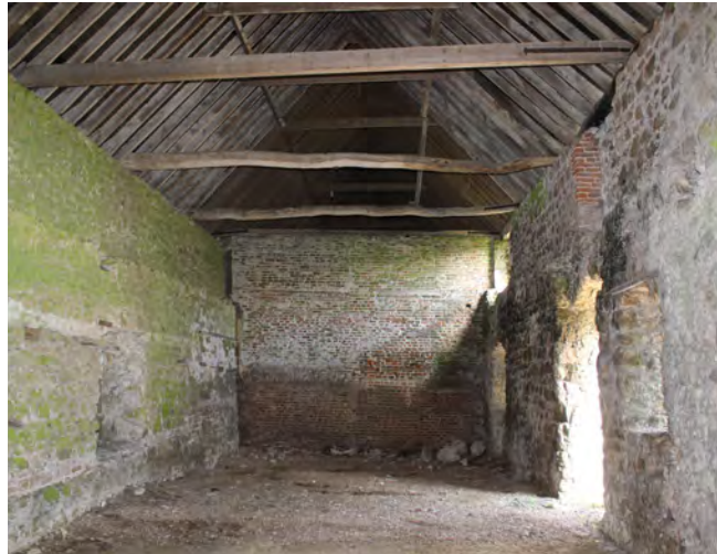
Figure 90: View of the west room looking east showing a later brick partition
