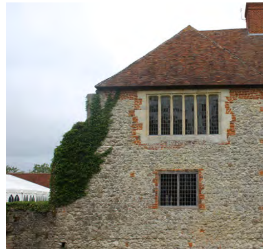
Figure 44: View of the east elevation of the main range which unlike the other ranges forms part of the 14th century ragstone curtain wall
