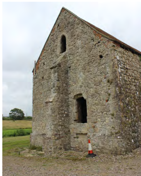
Figure 88: View of the west gable end showing the central buttress and lower and upper level openings
