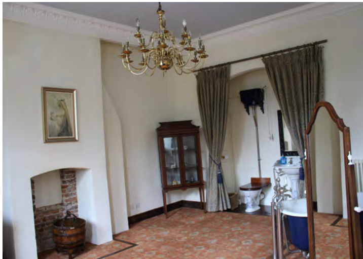
Figure 58: View of part of the bridal preparation suite at first floor showing modern corning poorly applied across the chimney breast
