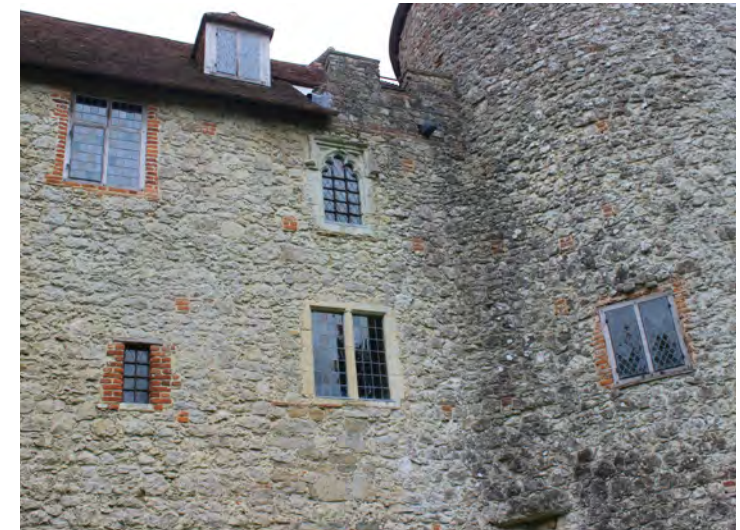
Figure 47: Detail of the east elevation of the rear wing showing several altered windows, as indicated by the later red brickwork, as well as an older mullioned window and a 14th century cinquefoil-headed light above
