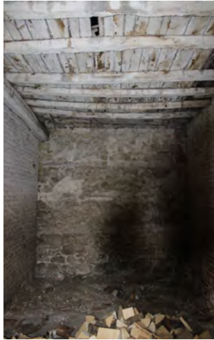
Figure 94: View of the small central room showing framing brick walls and a timber joist ceiling with a floor above
