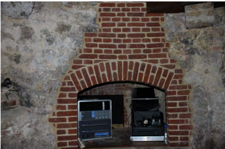
Figure 67: Former bread oven at ground floor level in the north-east tower (former bakehouse)
