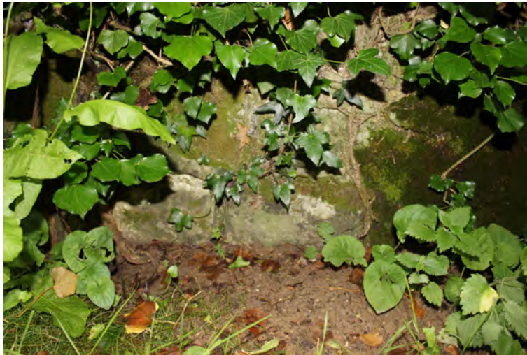
Figure 40: Detail of the masonry retaining wall separating the terrace from the moat
