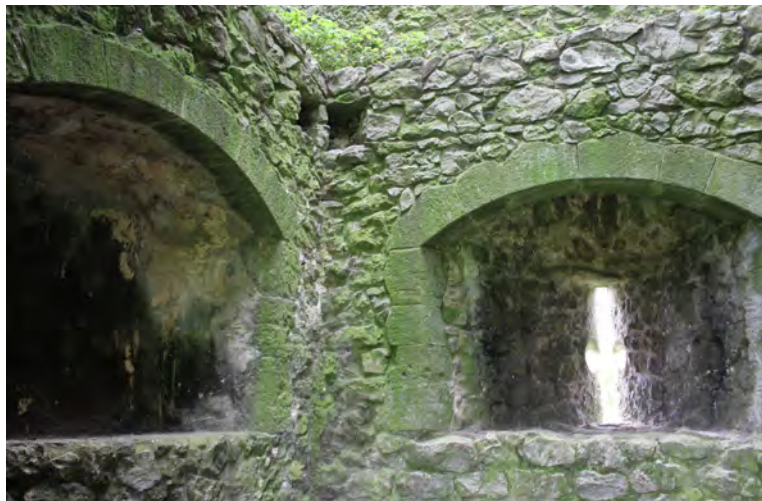
Figure 38: Internal view inside Rosamund's tower showing a slit window and a fireplace, both with dressed masonry surrounds
