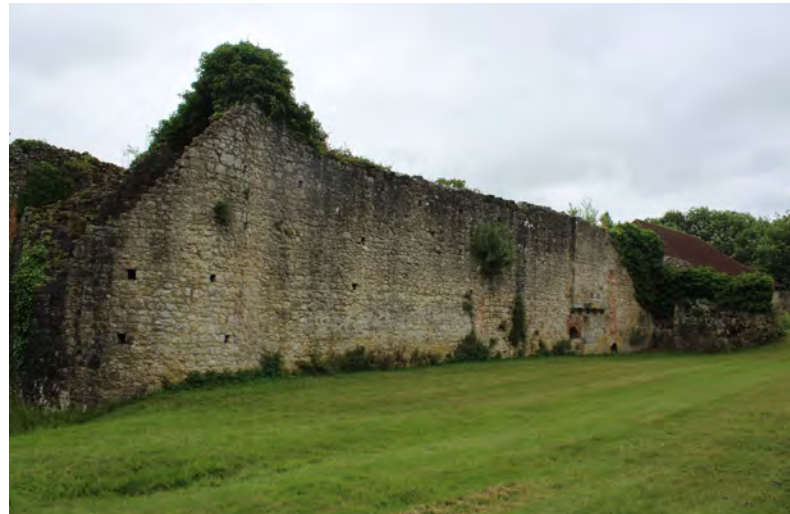
Figure 22: View of the north end of the west curtain wall looking south showing the north-west tower in the left foreground, the gatehouse in the right background and the infilled moat in front
