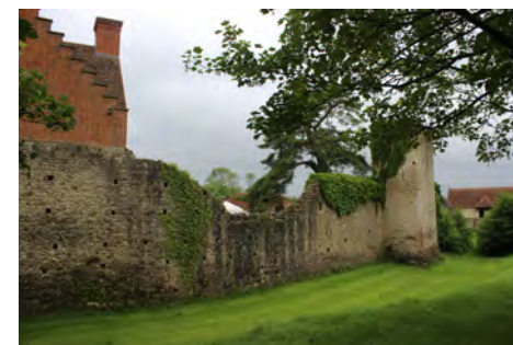
Figure 20: View of the north curtain wall looking west showing Rosamund's tower in the right background and the dry north arm of the moat in the foreground
