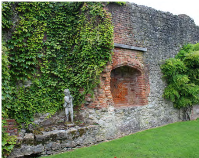
Figure 14: View of the west wall of the west range showing the red brick Tudor fireplace
