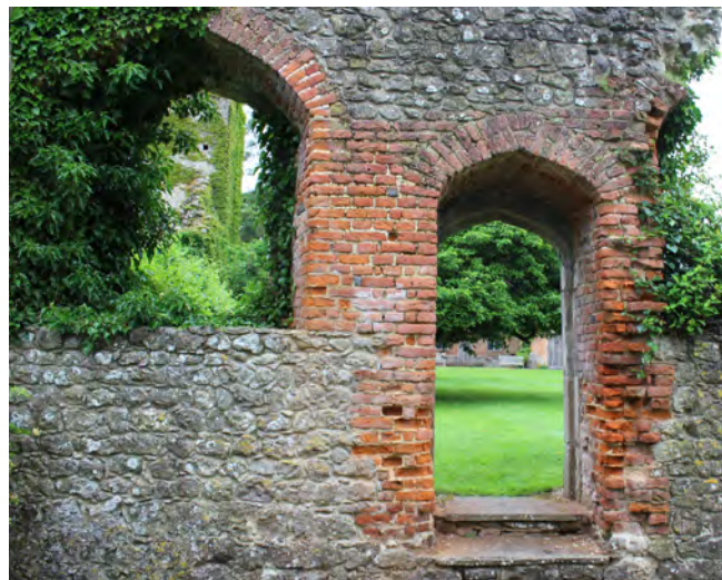
Figure 15: Red brick Tudor doorway and wide-splayed window opening in the west range
