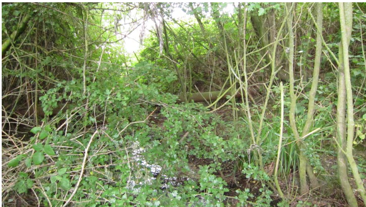
Figure 22 Disused existing metal rising main (220mm outside diameter) at the western edge of the racecourse lake
