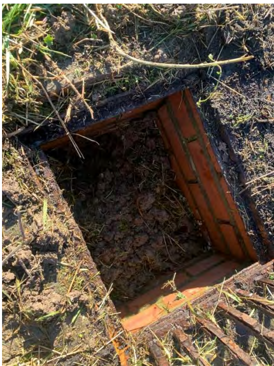
Figure 34 Blocked overflow catchpit chamber at the northern edge of the racecourse lake, near to the existing spillway
