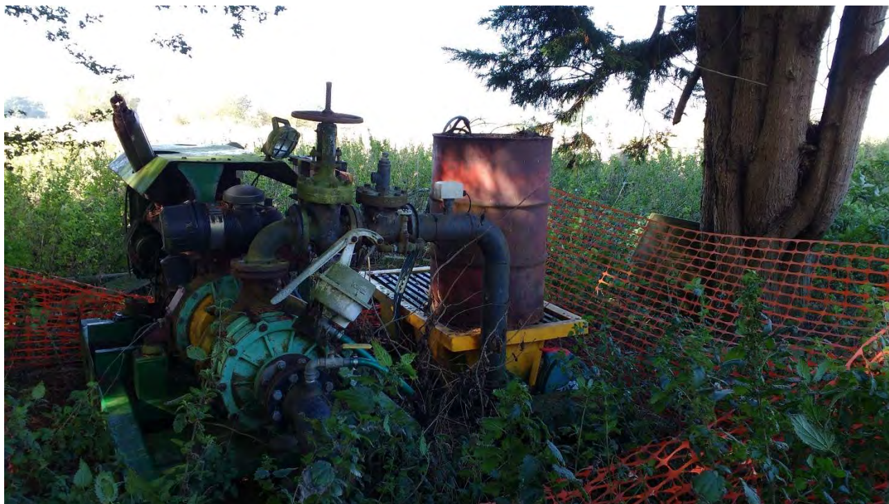
Figure 32 Disused second existing pump at the western edge of the racecourse lake
