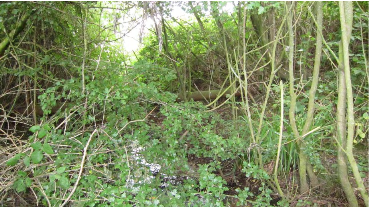
Figure 31 Disused existing metal rising main (220mm outside diameter) at the western edge of the racecourse lake
