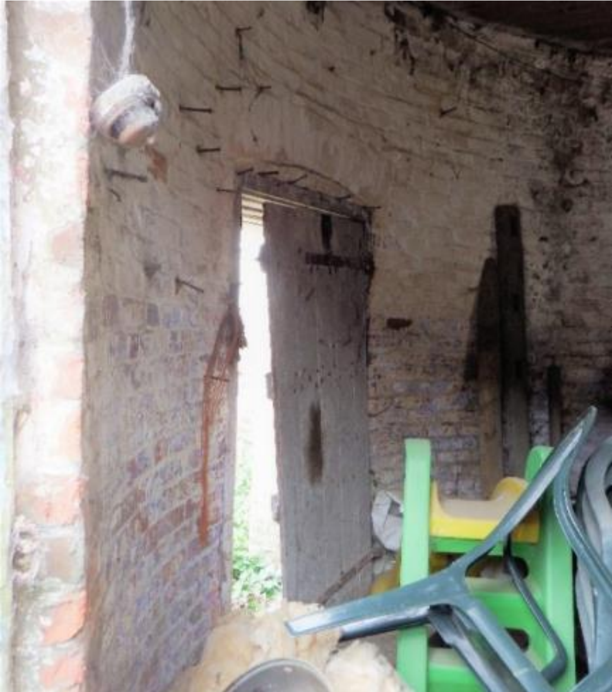
Plate 28: Internal door within oast house at Barrow Hill Farm leading to stable
