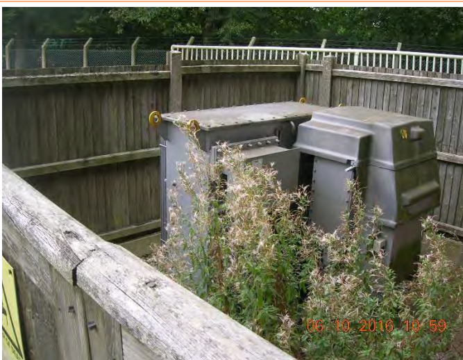
Photo 5: Electrical substation at racecourse
