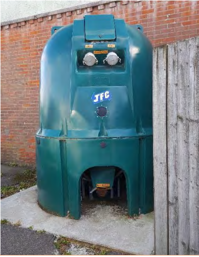
Photo 19: LPG tank at Newingreen
