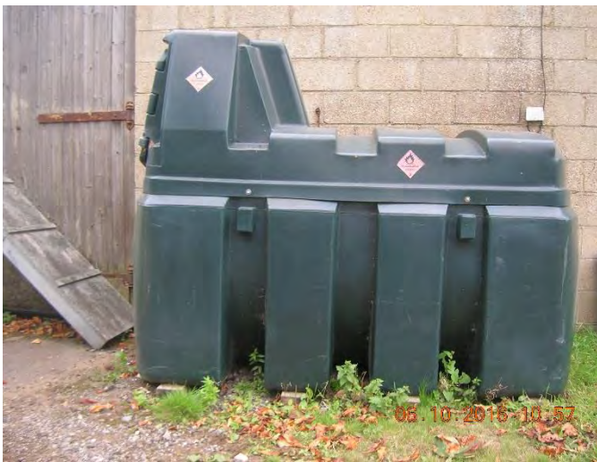
Photo 3: Bunded above ground fuel storage tank at racecourse
