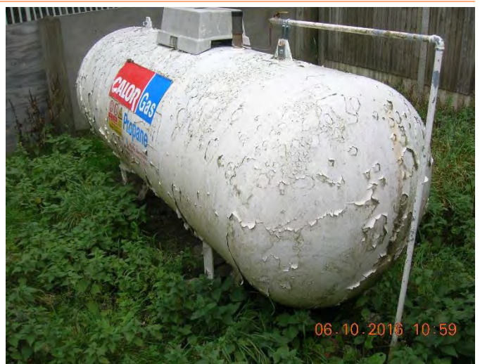
Photo 6: Above ground LPG storage tank at racecourse
