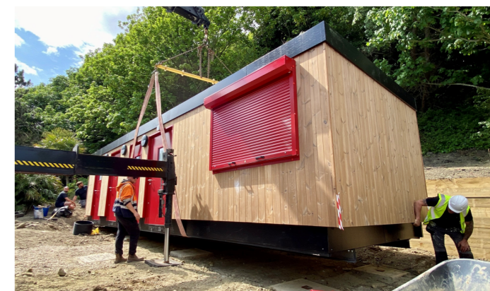
Installation of new solar powered facilities in the Lower Leas Coastal Park that opened in June 2023
