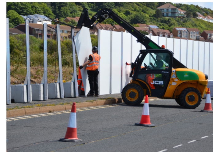
Removal of hoarding at Princes Parade site. A decision over the future of the site is due to be made after public consultation later in the year
